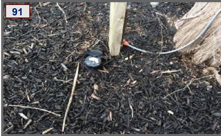
Water Meter Buried
