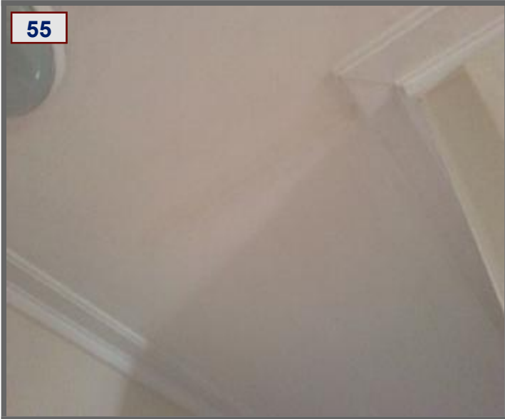
Cracked Plaster Ceilings
