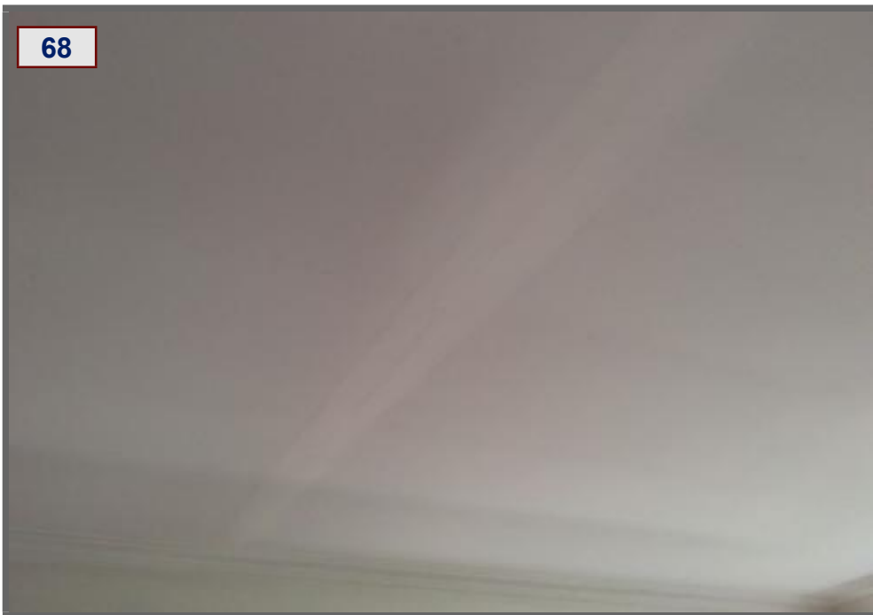
Cracked Plaster Ceiling
