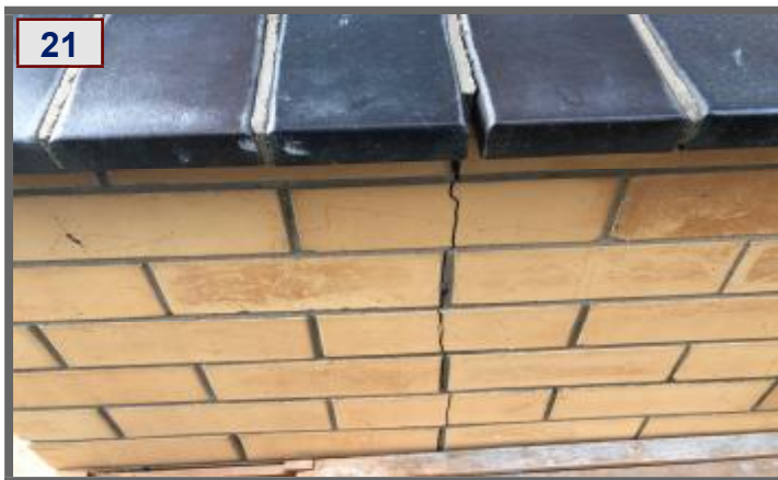
Brick Walls Cracked
