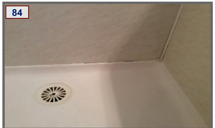
Sealant In Shower
