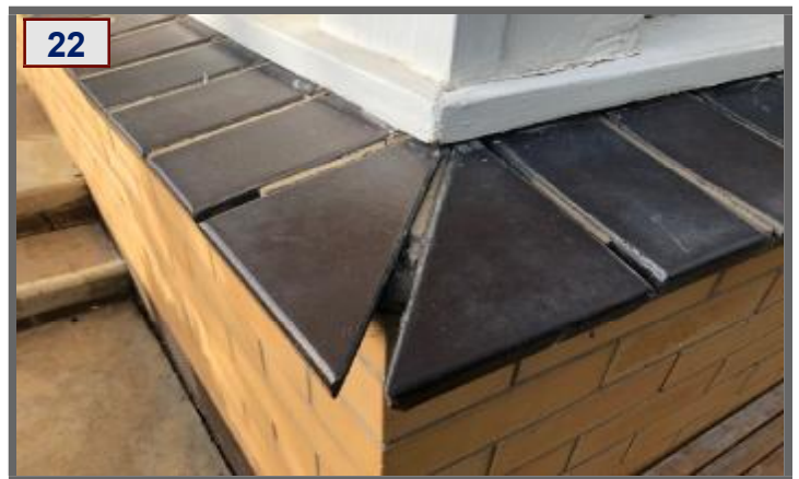
Sill Tiles Moved
