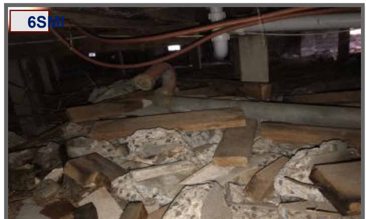
Debris Under Bathroom
