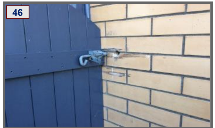
Gate Out Of Alignment
