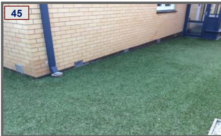
No Surface Drainage Installed
