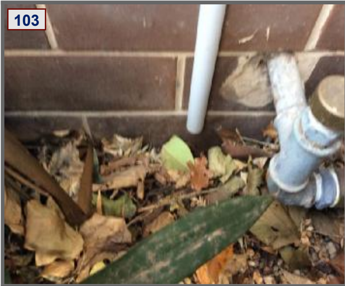
Condensation Drain Onto Ground
