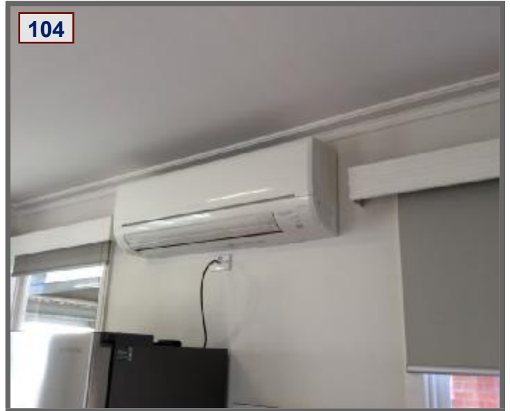
Split System Air Conditioner
