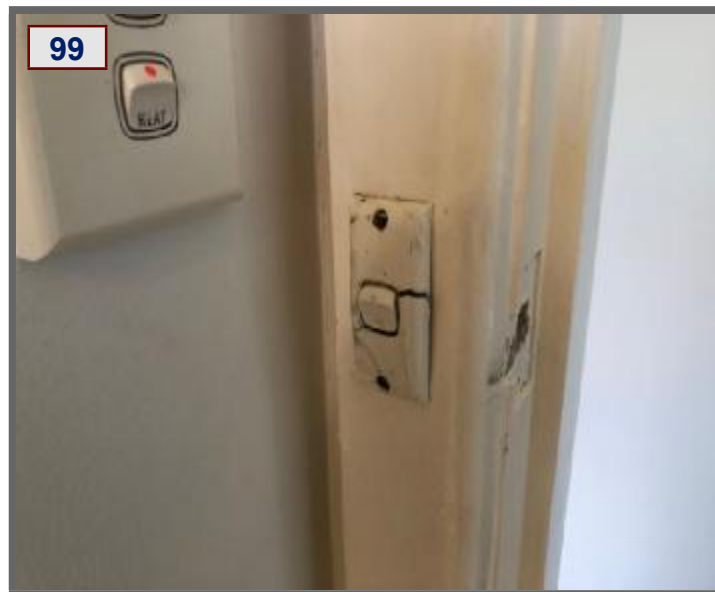
Light Switch Damaged
