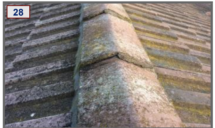
Tile Pointing Cracked
