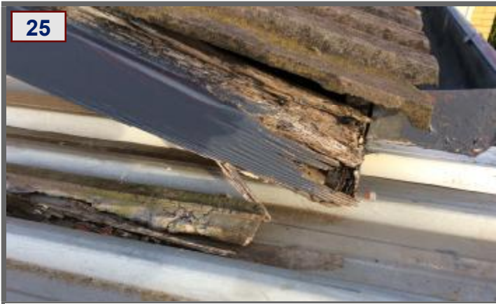
Fascia Boards Decayed
