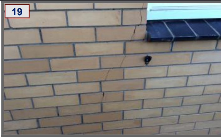
Brick Walls Cracked
