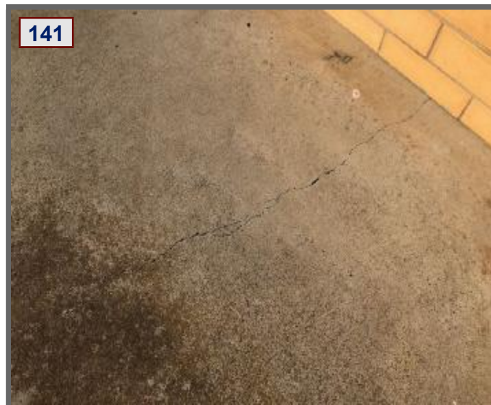
Cracked Concrete Paths And Balcony
