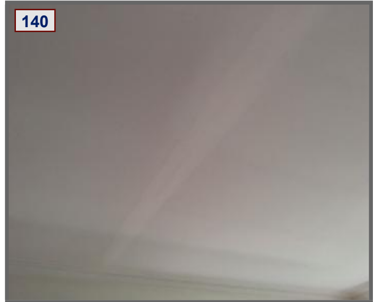
Cracked Plaster Ceilings In Several Locations
