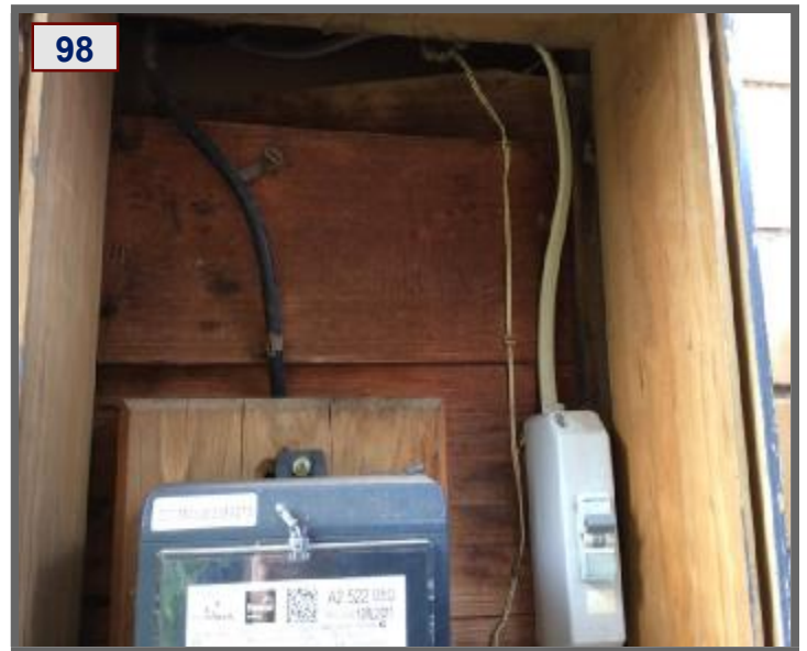
Meter Box Damaged
