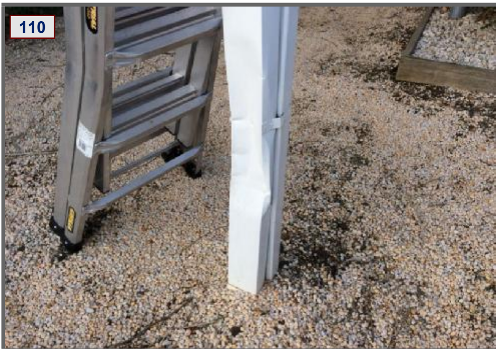
Down Pipe Damaged
