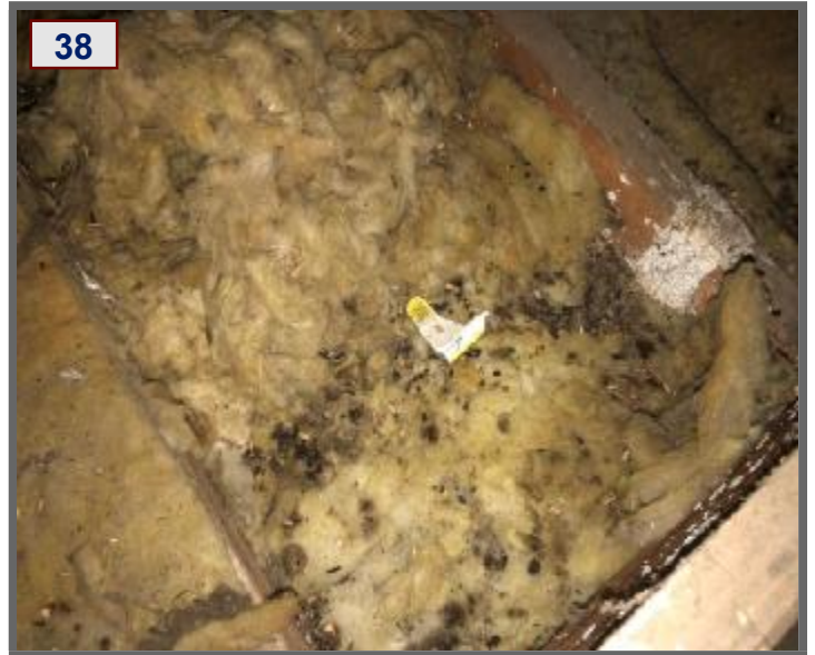
Evidence Of Rodents
