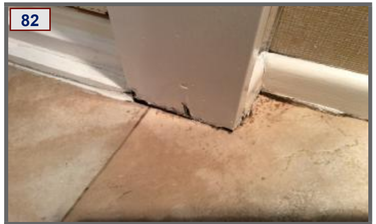
Leaking Shower And Decayed Timber
