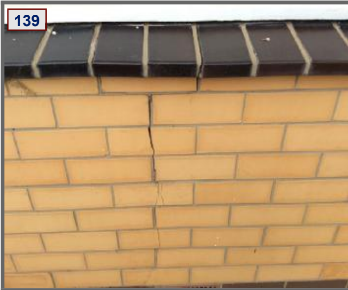
Cracked Brick Walls In Several Locations
