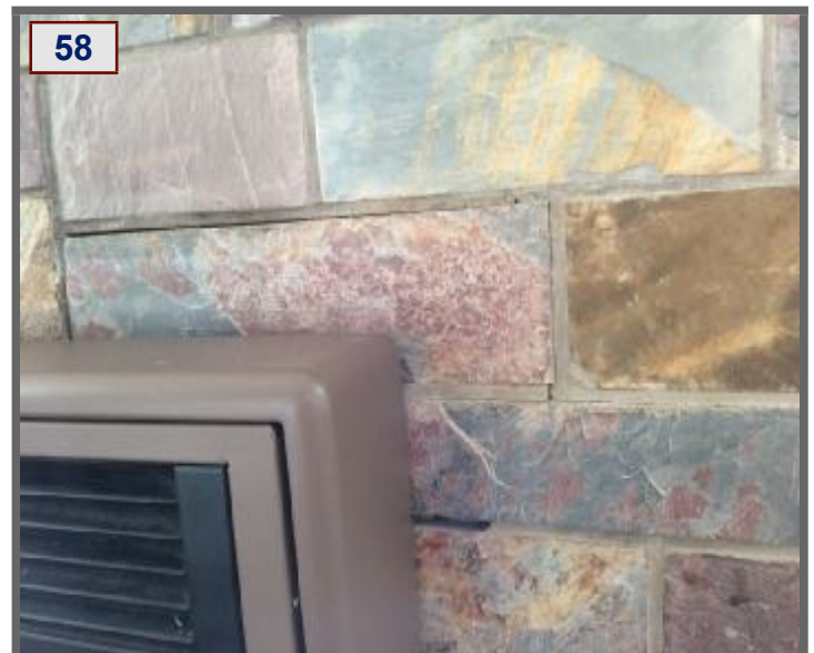
Cracked Tile Mantle
