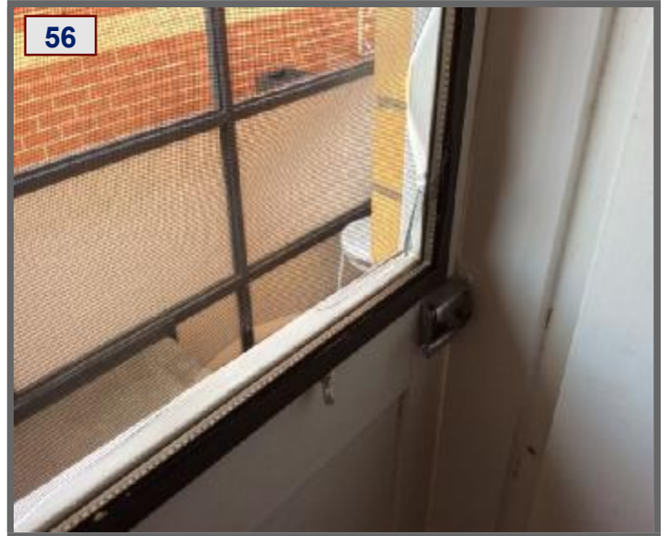
Damaged Insect Screens
