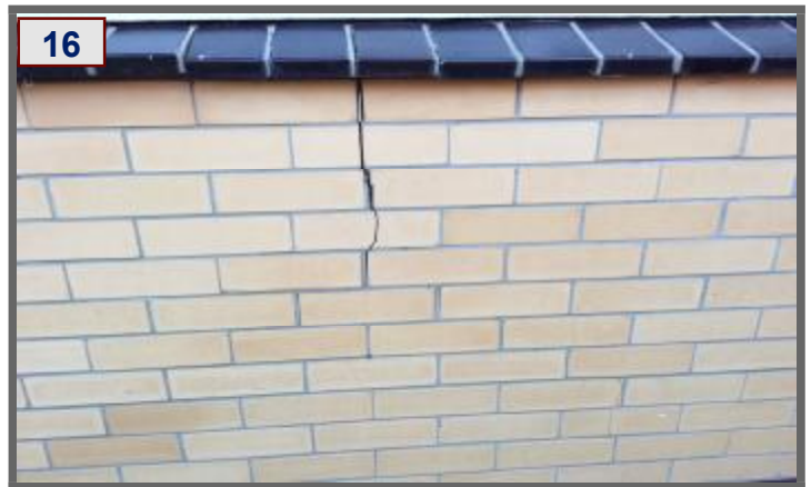
Brick Walls Cracked
