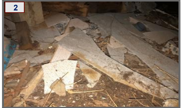
Cement Sheet Debris
