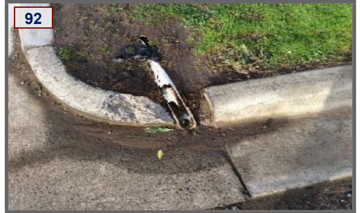
Storm Water Pipe Damaged
