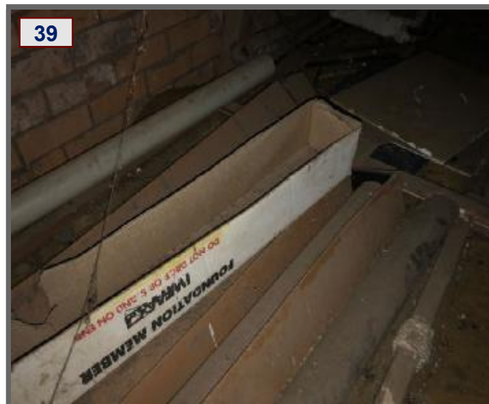
Debris On Ceiling
