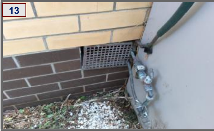
Brick Vent Loose
