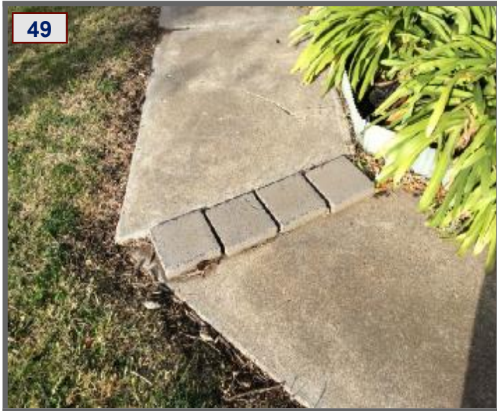
Paths Cracked And Displaced
