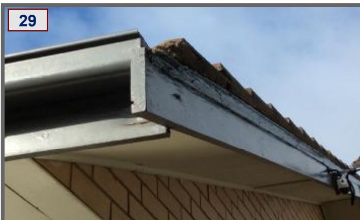
Fascia Boards Decayed
