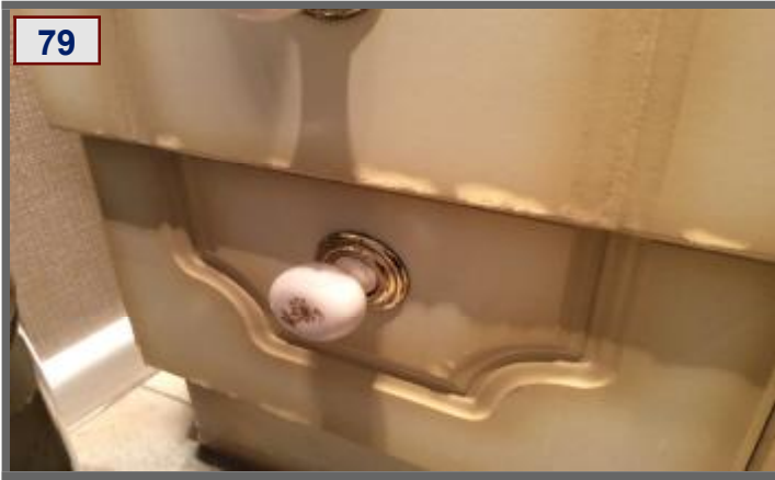
Water Damaged Vanity
