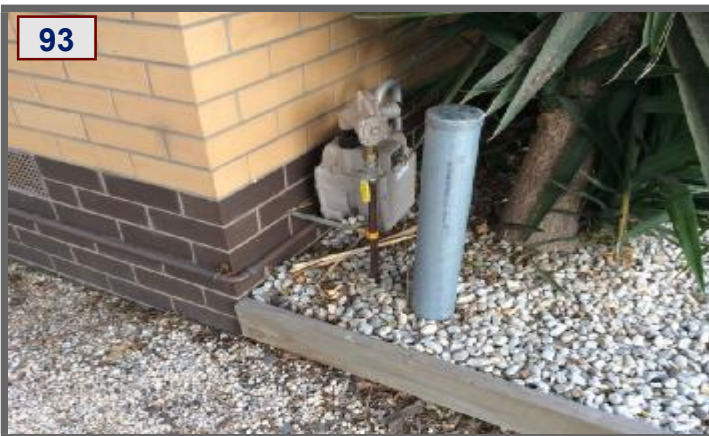
Gas Meter Location
