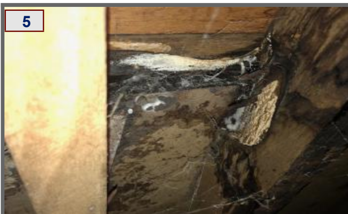
Floor Under Shower Damaged
