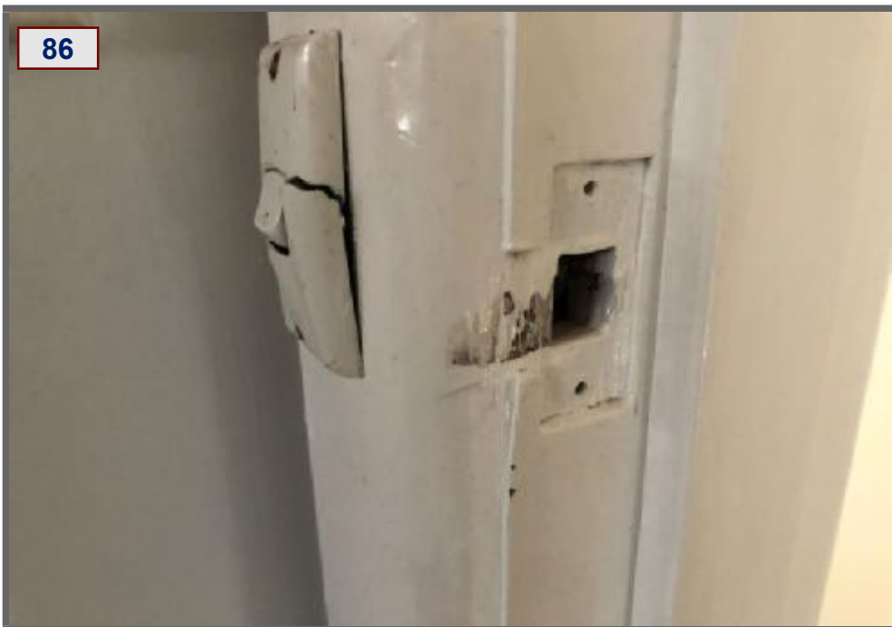
Door Strike Missing
