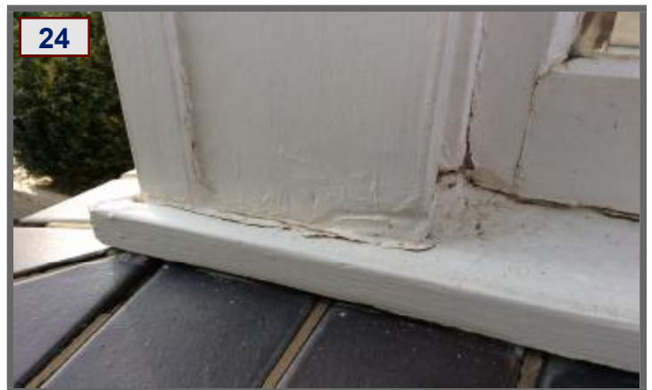
Windows Decayed And Repaired
