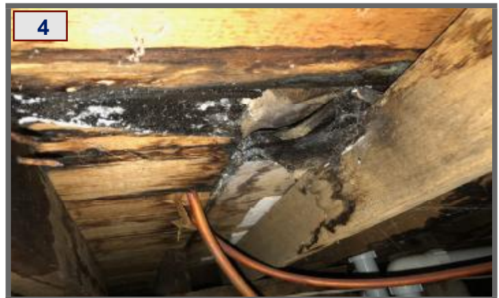
Floor Under Shower Damaged
