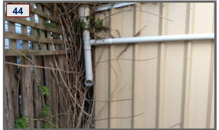
No Storm Water Connected On Shed
