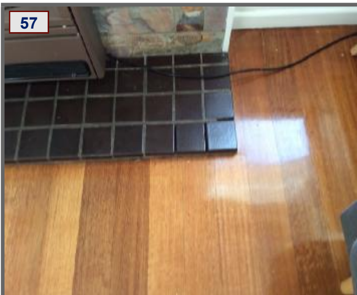
Damaged Tiled Hearth
